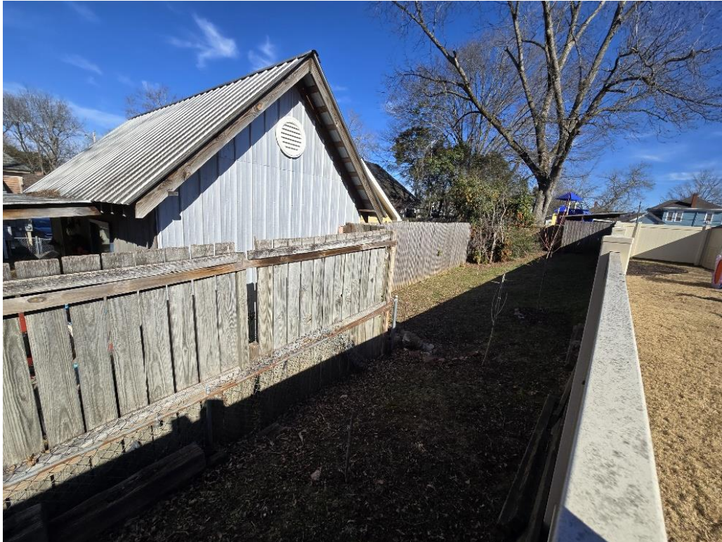
View of area in question between Church property (to the right) and neighbors (to the left)
