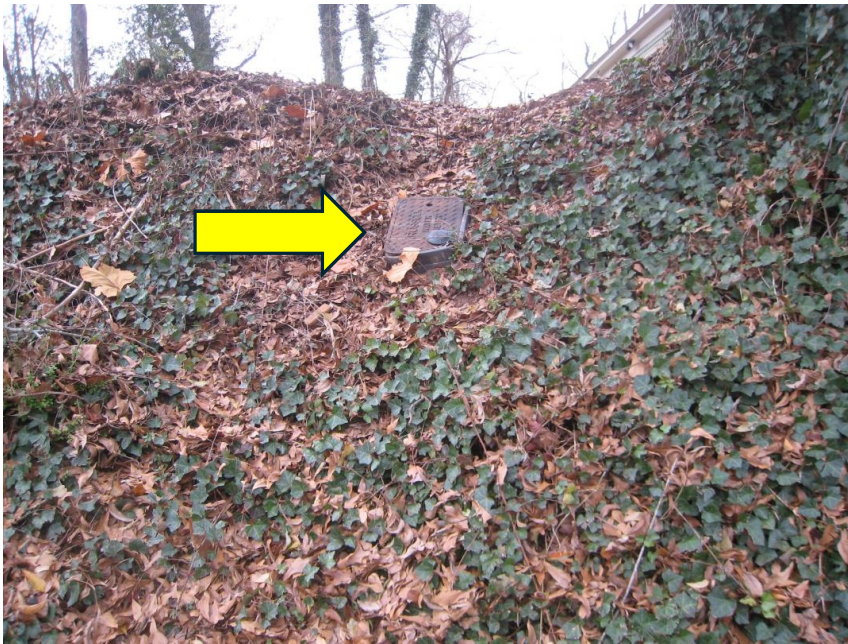
Alternate view of steep slope in front of subject property along East Broad Street (note the water meter's location – see arrow)
