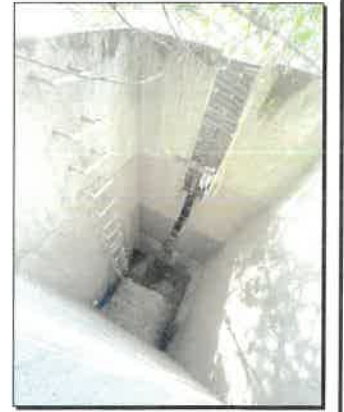
② INSIDE NORTH WESTERN OCS
