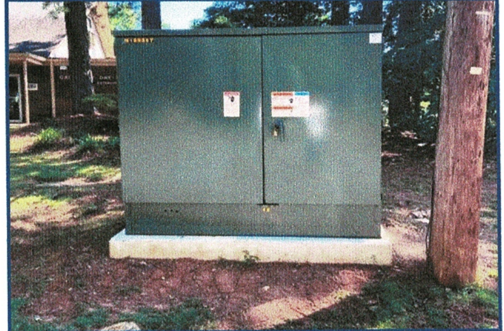
Three Phase Transformer .16
